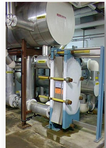
Plate-and-frame liquid chiller
