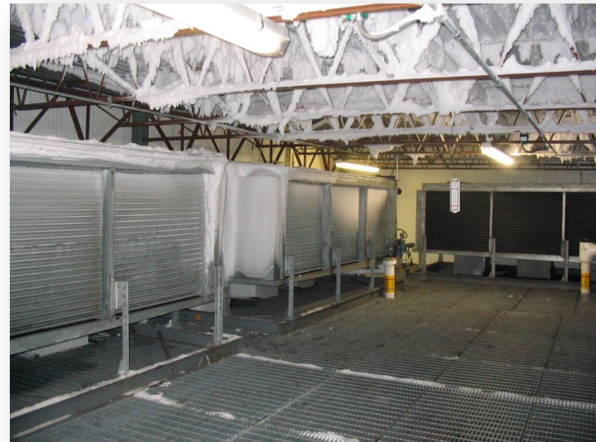
Penthouse evaporator in a freezer
