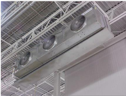
Ceiling-hung evaporator in a dock area
