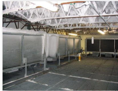
Penthouse evaporator in a freezer
