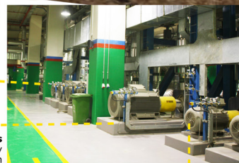
Production Pumps 5 on Duty + 1 Standby Total flow: 7,140 m 3 /h
