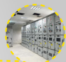
Low Voltage and Medium Voltage Rooms
