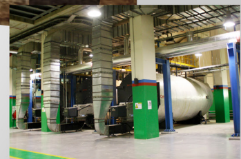
Boilers 6 of 16,000kW 1 of 5,000kW Dual Fuel & Gas Burners Minimum Efficiency= 92%
